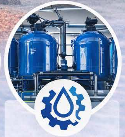
Endüstriyel Arıtma Industrial Water Treatment Filtrasyon & Su Arıtma Filtration & Water Purification
